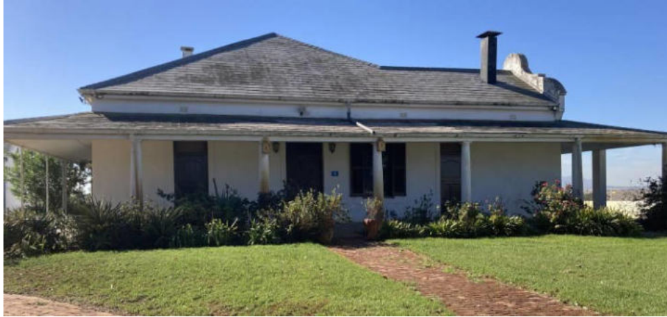
Figure 22: The roof is of asbestos cement shingles and the veranda roof is supported on steel pipe columns, Pre-cast concrete columns and brick columns
