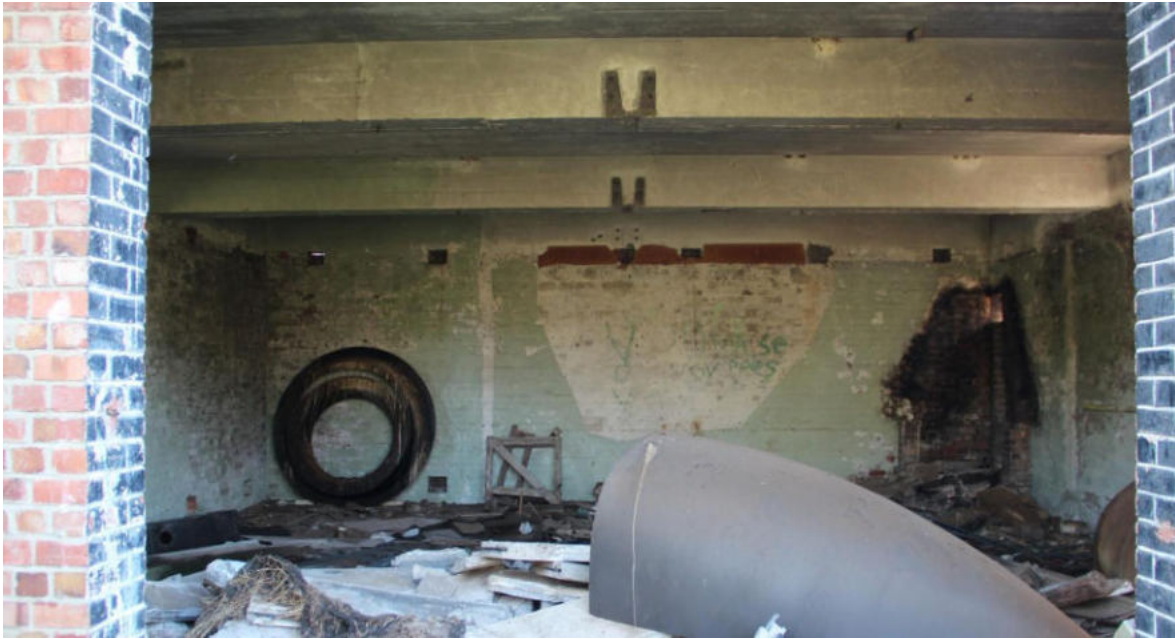
Illustration 17: The interior of the Workshop showing the evidence of a gantry and a forge (Structure #2, SSTownsend, 15 June 2020)
