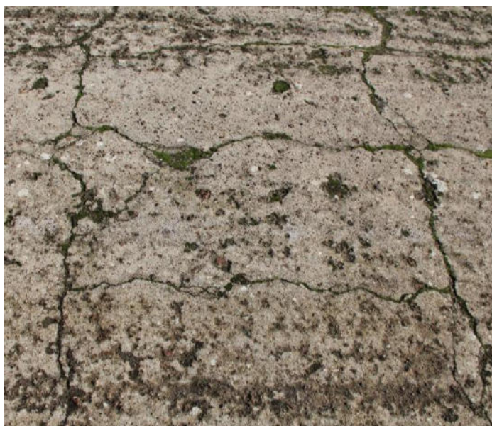
Illustration 20: A 500mm square sample of the cracked concrete (SSTownsend, 15 June 2020)
