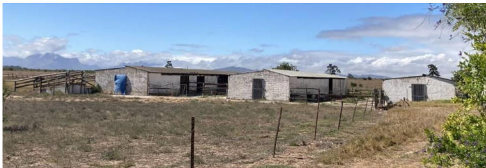
Figure 17: Stabling of concrete blocks with roofs of asbestos sheeting
