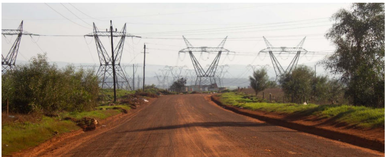
Figure 41: Site photograph demonstrating the intensity of visual clutter as a result of the Eskom power lines where these cross Canary Street near Fisantekraal (Smit, 2021)
