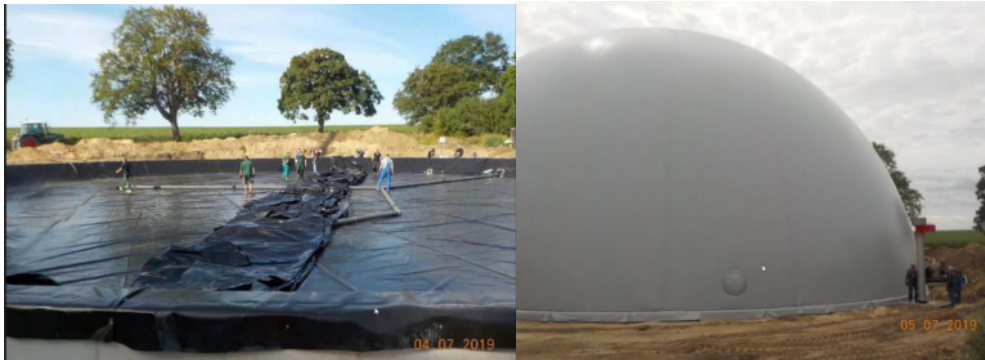
Biogas Bladder Storage
