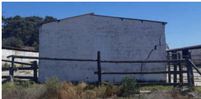
Figure 56: Corner down type crack possibly related to potentially expansive nature of subsoils; stable structure located between TP18 and TP15.
