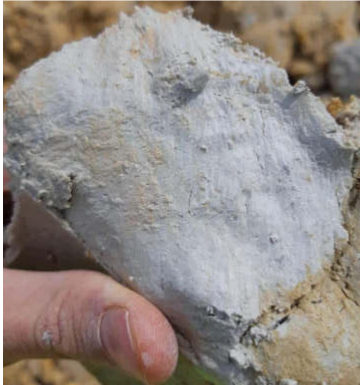
Figure 55: TP44 – Close-up of slightly smoothed/slickensided surface of residual material encountered in trial pit.
