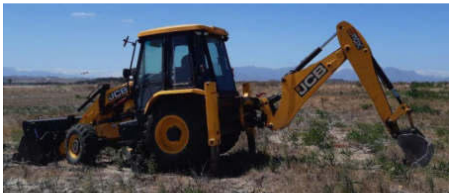
Figure 60: View of JCB 3DX Super Tractor Loader Backhoe excavating a trial pit near the central portion of the site.
