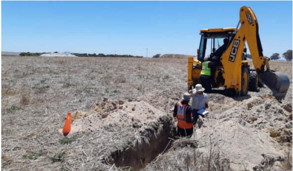
Figure 44: TP21 – GEOSS team conducting DCP test beneath nodular ferricrete horizon. White clay-silt Corrobrick material pictured in the background.
