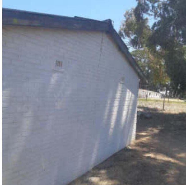
Figure 57: Vertical crack possibly related to potentially expansive nature of subsoils; storage structure located between TP18 and TP15.
