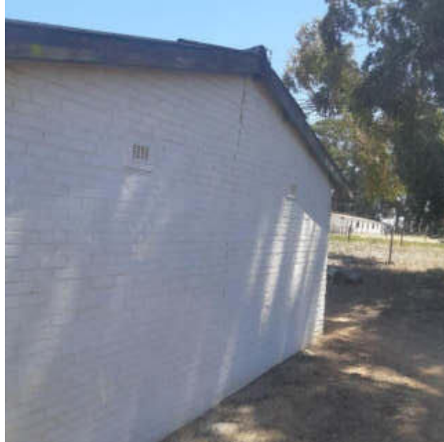
Figure 57: Vertical crack possibly related to potentially expansive nature of subsoils; storage structure located between TP18 and TP15.
