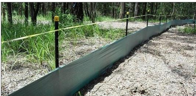
Figure 159: Example of a barrier fence used to demarcate the no -go area around the freshwater ecosystems and the 15m construction conservation buffer (FEN: Sept 2024)
