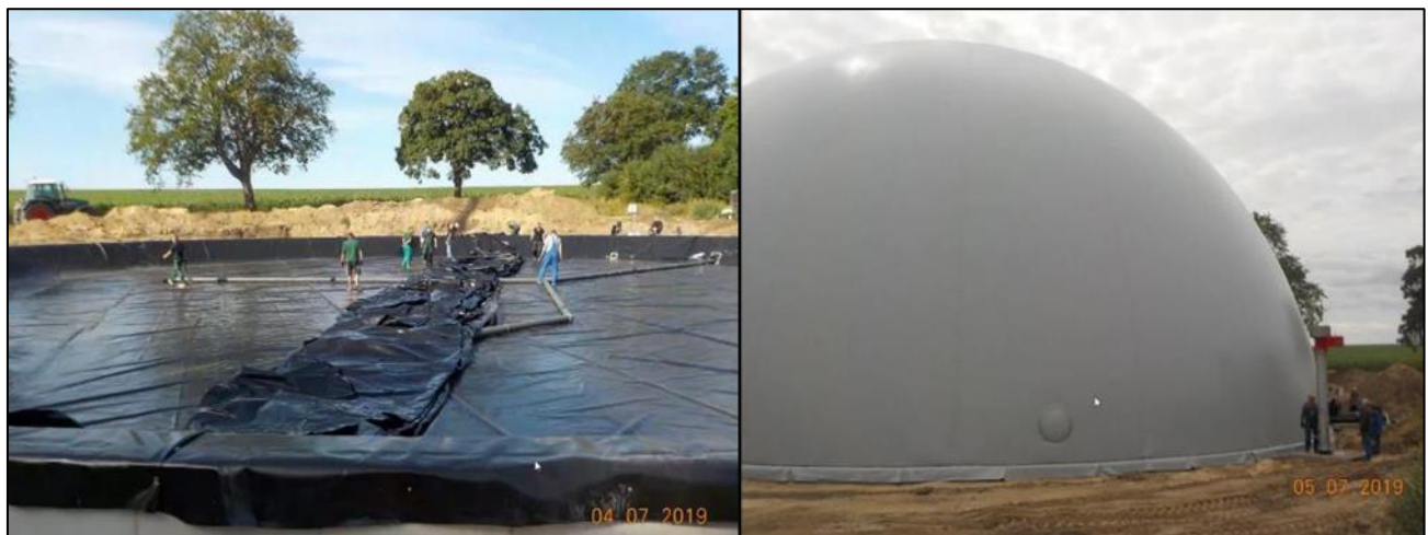
Figure 37: Example of Biogas Bladder Storage (SANDS, Electrical Bulk Services Report, Oct 2023)
