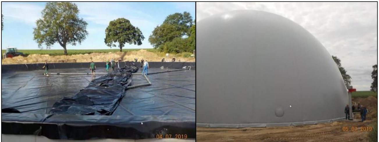
Figure 43: Example of Biogas Bladder Storage (SANDS, Electrical Bulk Services Report, Oct 2023)
