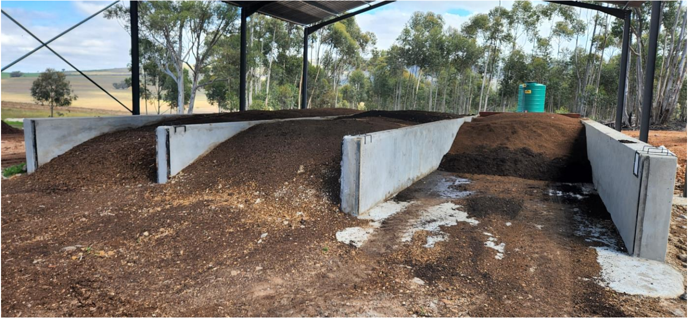
Figure 3: Static concrete composting bunkers on the Remainder (RE) of farm Grootvlei 225, Caledon.
