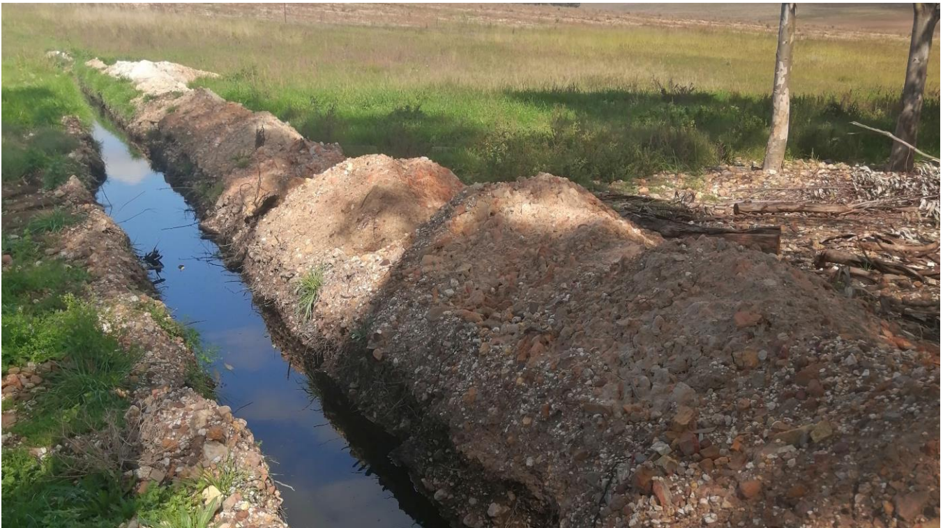
Figure 4: Stormwater control channel west of the composting facility on the Remainder (RE) of farm Grootvlei 225, Caledon.
