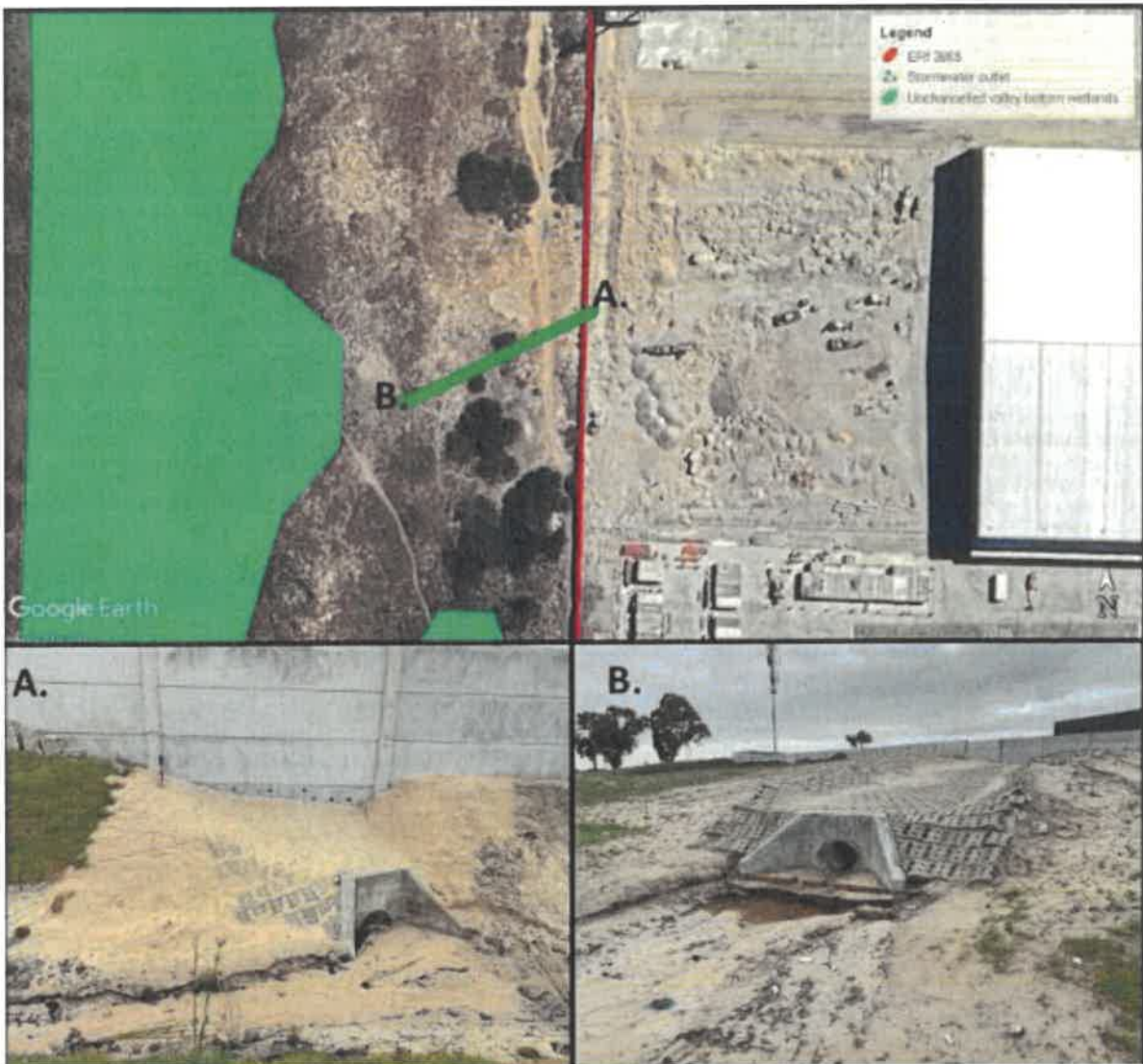
FIGURE 6: A GOOGLE EARTH SATELLITE IMAGE OF THE WESTERN BOUNDARY OF THE SITE SHOWING THE LOCATION OF THE STORMWATER OUTLET FROM THE ATTENUATION POND, A) THE INLET TO THE STORMWATER OUTLET PIPE WITHIN THE ATTENUATION POND AND B) THE OUTLET FROM OF THE STORMWATER OUTLET INTO THE KUILS RIVER CORRIDOR, SHOWING EROSION DOWNSTREAM OF THE OUTLET (AQUATIC RISK ASSESSMENT REPORT FOR THE PROPOSED ABSTRACTION OF GROUNDWATER AT THE ACKERMAN'S DISTRIBUTION CENTRE ON ERF 3865, HAGLEY, STUART BARROW (SEPTEMBER 2024))
