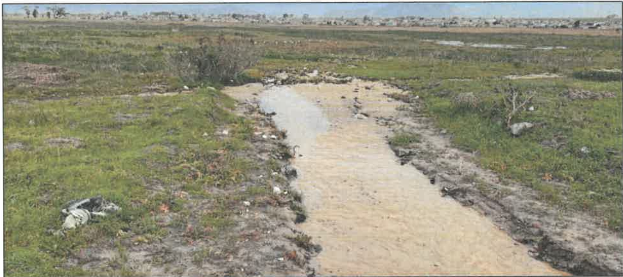
FIGURE 3: SEDIMENT DEPOSITION OCCURRING WITHIN THE KUILS RIVER CORRIDOR AT THE STORMWATER OUTLET.
