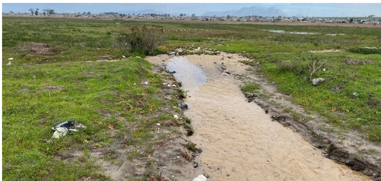
Figure 15. Sediment deposition occurring within the Kuils River corridor at the stormwater outlet.
