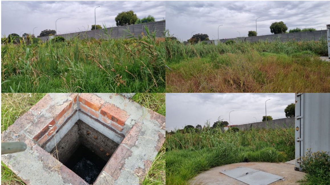
Figure 3. Images of Phragmites beds (top) that has formed surrounding the stormwater drainage system (bottom).
