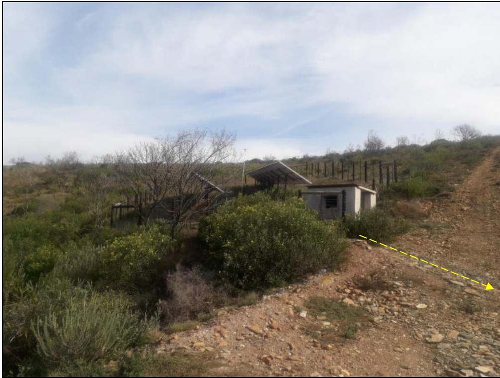
Photo 30: Larger dam – pump station and solar panels. Note swale taking stormwater downstream from pumpstation area (indicated by yellow dotted arrow to indicate flow)
