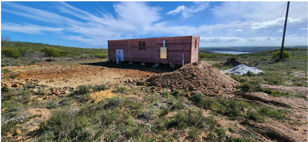
Photo 4: View of the cleared area around the new caretakers cottage located in the southern portion of the property, adjacent to the farms internal access road (facing north)
