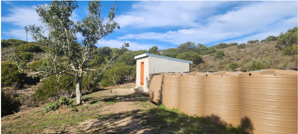
Photo 8: View of a portion of the cleared area around the main dwelling where a new pumproom has been constructed and additional water tanks have been installed.
