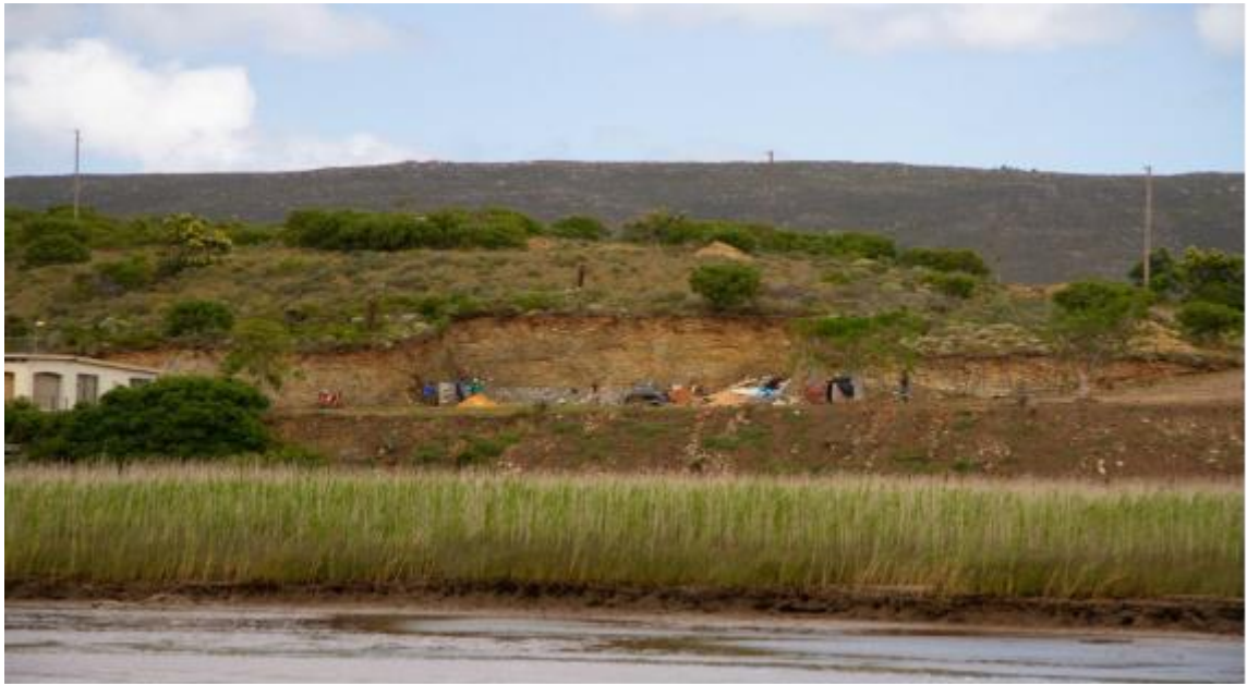
Photo 1: View of the expansion area adjacent to the existing dwelling where there was clearing of indigenous vegetation and excavation into the slope.
