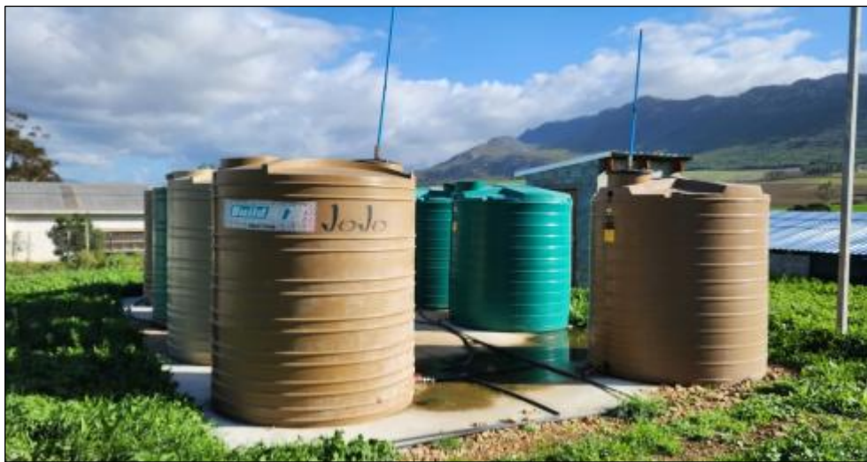
Figure 7: Jojo tanks used to store water.
