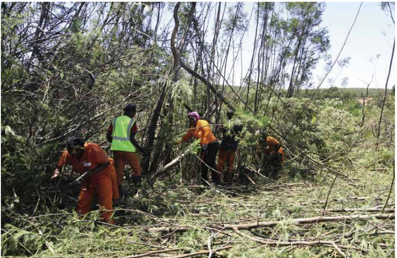
A clearing team in the Vyeboom Wetland near Theewaterskloof Dam in the Western Cape stacking cut black wattle.
