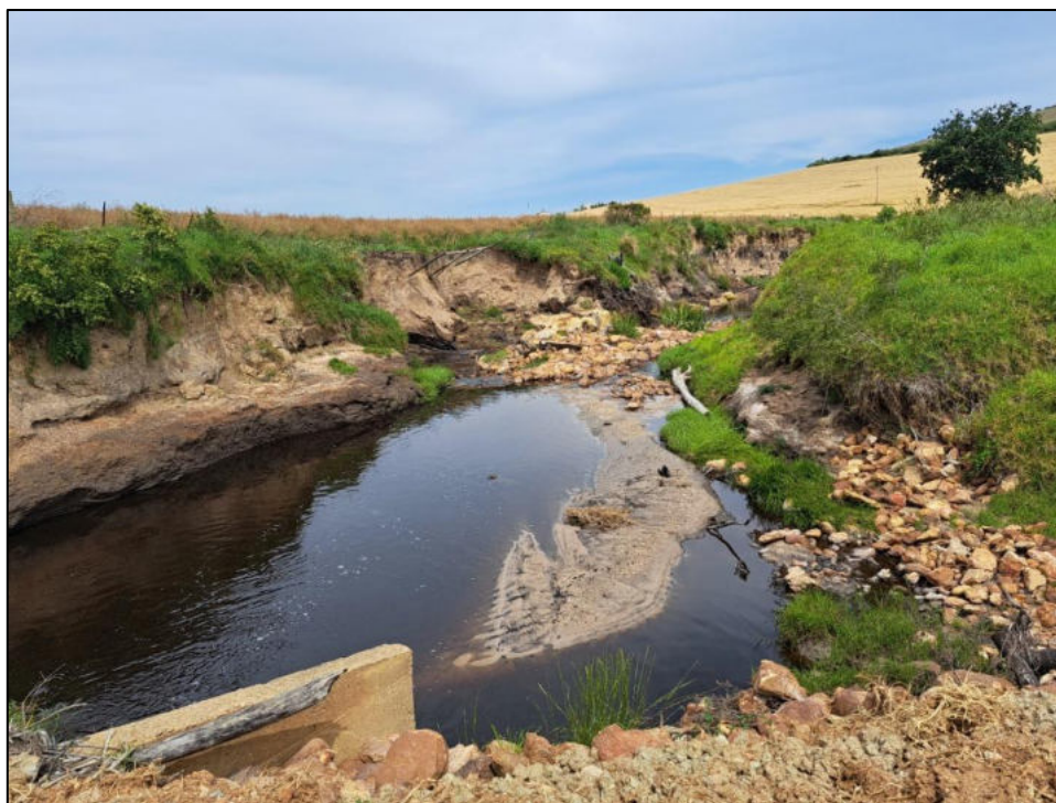
Figure 7: Photograph showing severe streambank and channel erosion downstream of Portion 3 of Farm 186.
