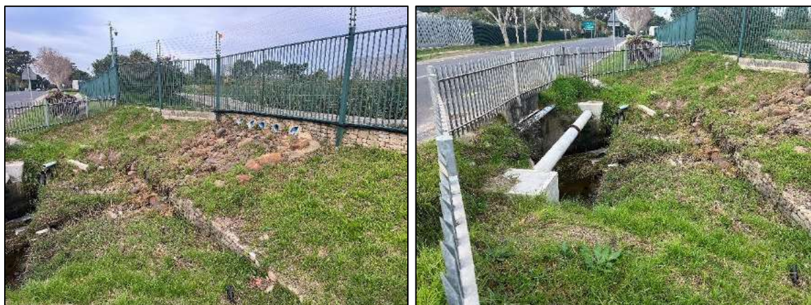
Figure 8: The Tokai Road crossing at the outfall of the main watercourse that leaves the study area (the golf estate). This structure does not allow for freedom of movement for fish from downstream within the catchment.
